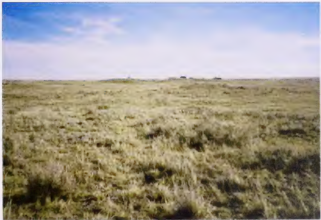
Photo 30 No-strip pipeline construction can reduce the impact to the native prairie vegetation.
